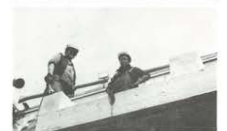
Looking up at carpenters Murray Dunphy and Harry Samm, replacing re-entry deck at #3 Woodroom. The old one had just about reached its allotted time.
