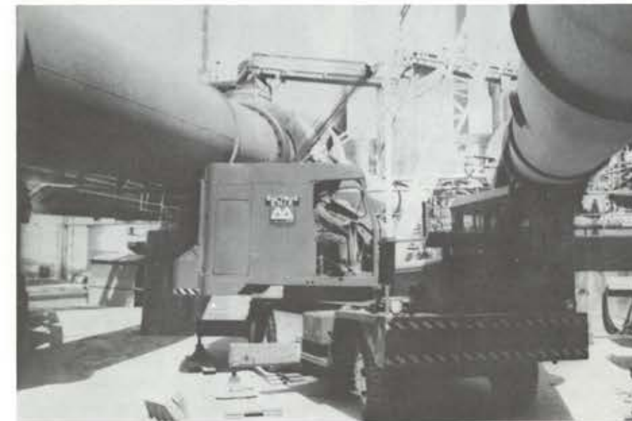
That's Jim Mardon and his mobile Bucyrus-Erie, working with Project Crew 73, hoisting the old top from the lime mud washer tank. Getting the big 25-ton crane into position took a bit of manoeuvring, and involved dismantling the 60-foot boom and re-assembling it again once the machine was wedged inside the re-caust area.
