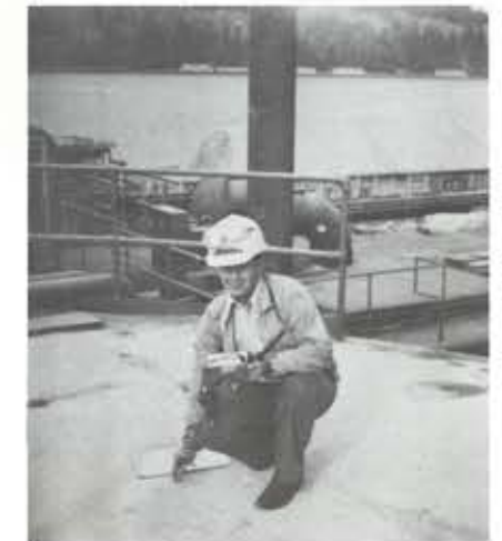
Maintenance Technologist Doug McLaren checking the steel top of a large storage tank. The instrument Doug is using is an ultrasonic thickness tester, so accurate that it can measure the thickness of a metal plate to a thousandth of an inch.
