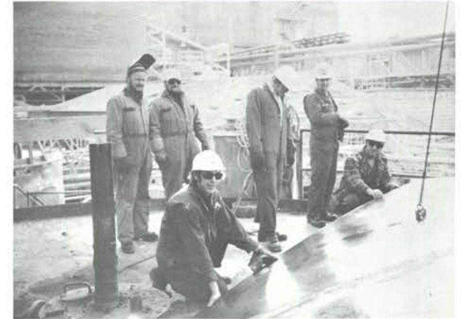
Project Crew 73, fitting a section of the new steel top of the lime mud washer tank. The four crewmen standing are Welders Bruce McKinley and Larry Bishop, and Millwrights Wayne Dulmage and Ken Mitrenga. Kneeling, closest to the camera, is Millwright Larry Paul, and furthest away on the extreme right is Lead Hand Ken Lesosky.
